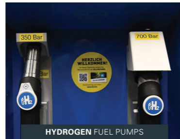
HYDROGEN FUEL PUMPS
